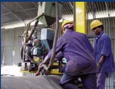
Pipes and Process Equipment, India rising
